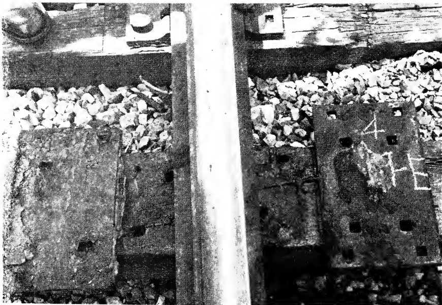
FIG. 17. North Portion Section 4, 13-in Bird Vinyl Tie Pad. Coated. After 25-months' Service in the Inner Rail of the Long 4-1/2° Curve.
